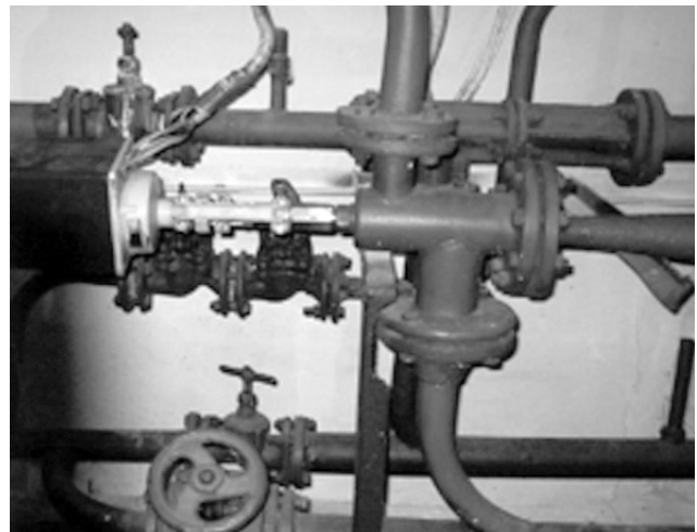
Typical heat substation with hydroelevator as a heat control at building level.
